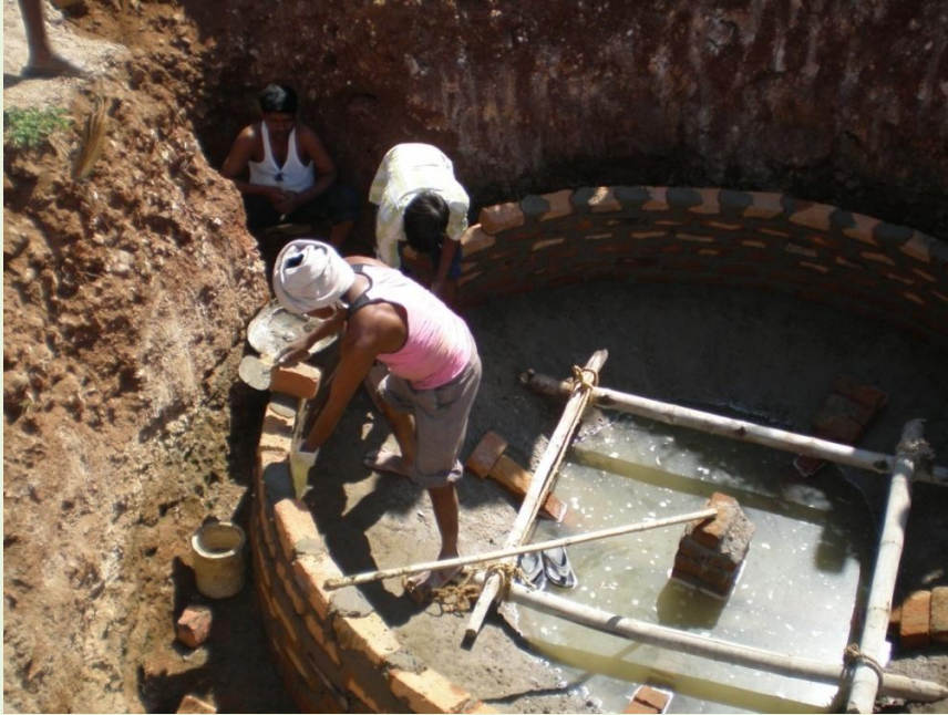
Deenabandhu Biogas plant
