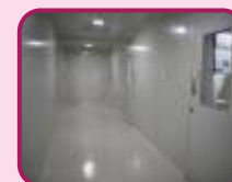
Clean Room Facility
